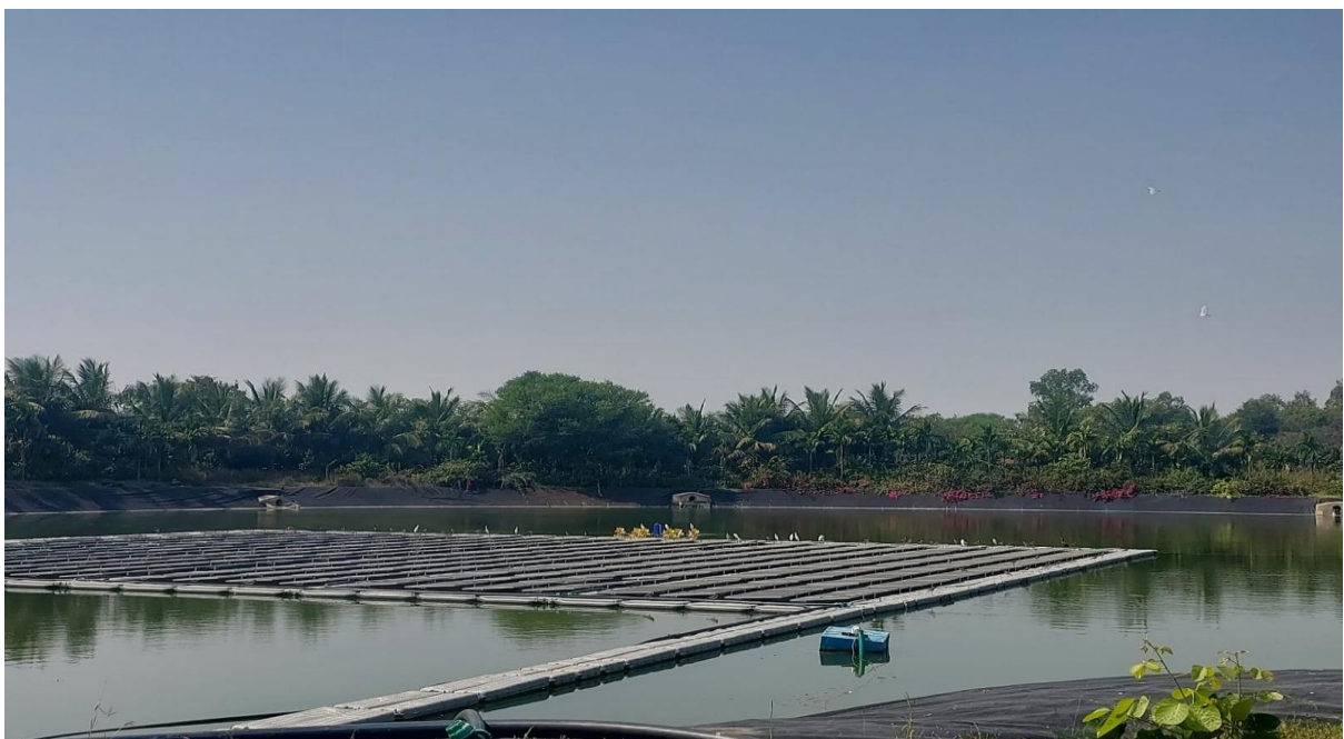
Site visit to Climate-Resilient Water Management Facility with Floating Solar Infrastructure at Kanha Shanti Vanam, Hyderabad
